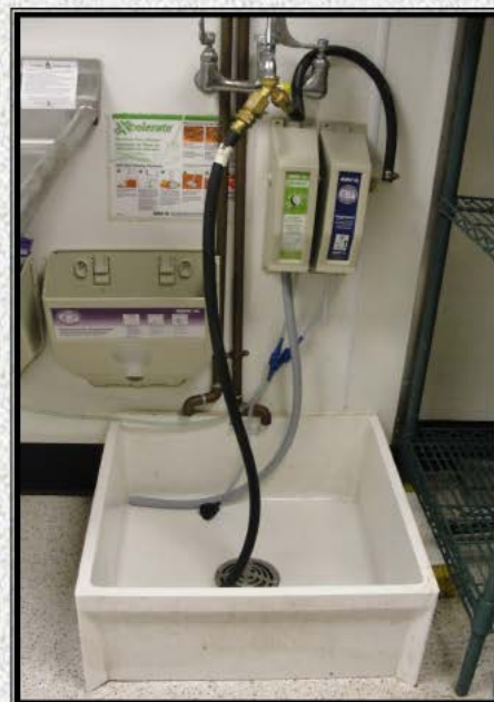
CURBED CLEANING FACILITY
